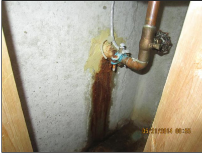
16.0 Item 1(Picture) Leak At Main Water Shutoff
