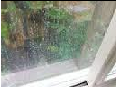
11.5 Item 1(Picture) Master Bedroom Window Condensation
