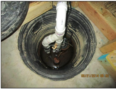
15.5 Item 1(Picture) Sump Pump
