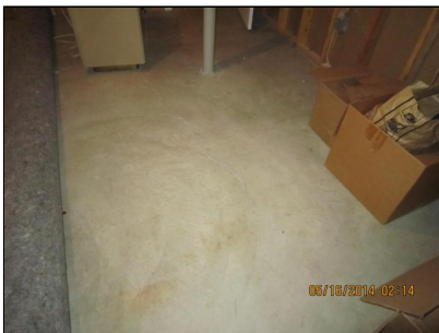
15.3 Item 1(Picture) Common Crack Basement Slab
